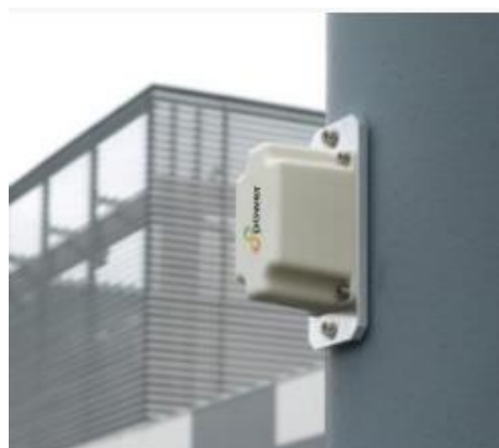
Sensor installed on bridge
